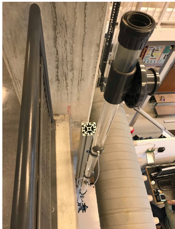
Figure 4. 7 Inlet at the top side of the pipe
