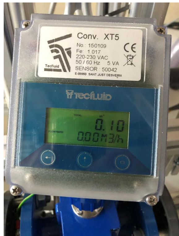
Figure 3.21. Flowmeter after test.
