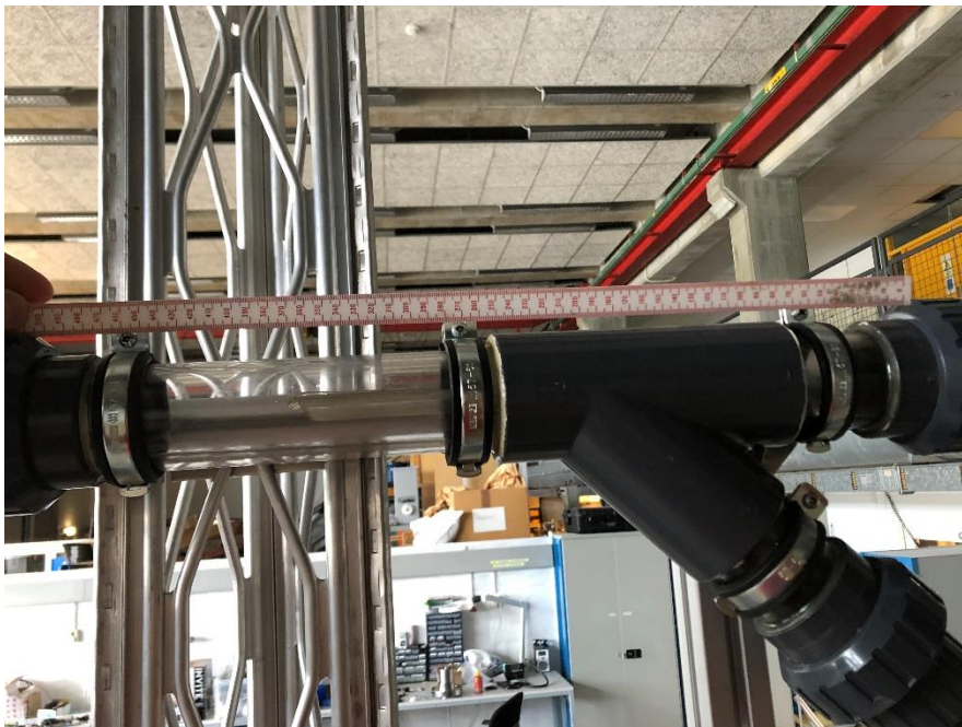
Picture 23. Mixing Unit.
