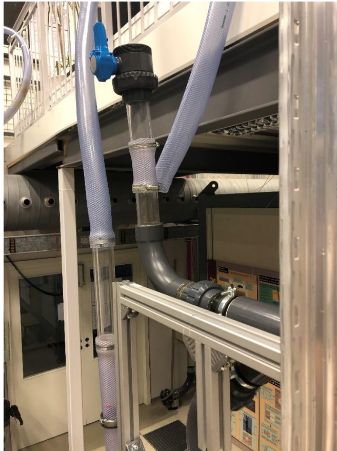
Picture 22. Vertical pipe.
