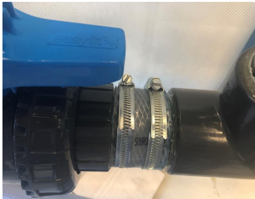
Figure 3.16. The weak point with fairly loose hose rings.
