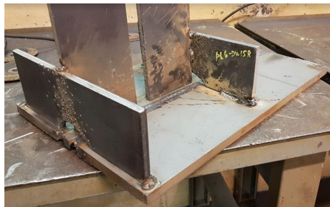
(g) Cracked tack weld was discovered after finished weld operation.
