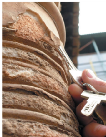
Figure 1- Marble displaying flakes and granular disintegration in Granada, Spain (Luque et al., 2011)
