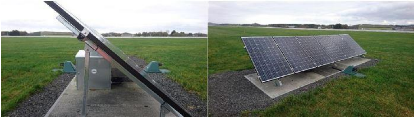
Figure 15 Solar Panels at Stavanger Airport (Avinor AS, 2019) as in Scenario 1.
