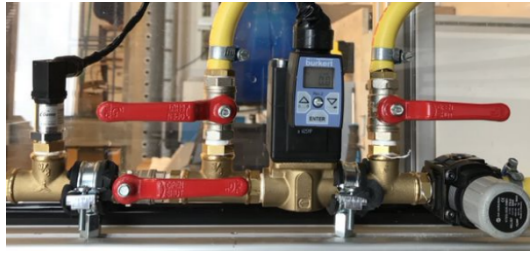
Figure 22: Picture of the manifold mounted inside the rig
