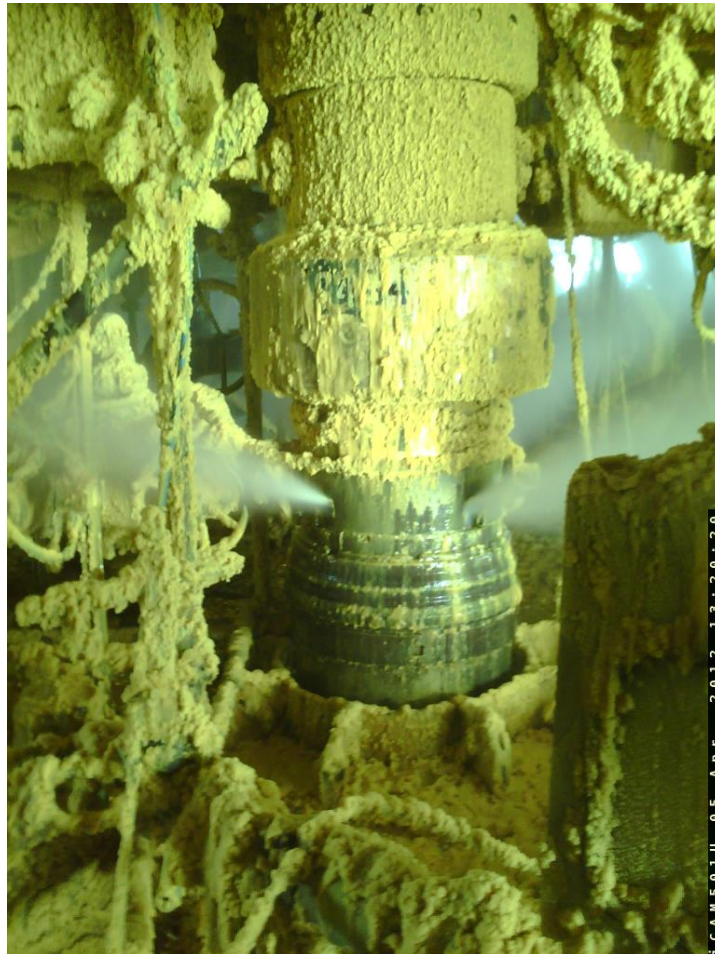
Fig. 14 - Surface wellhead D annulus leak, Elgin G4 well (Total E&P UK Ltd 2013)
