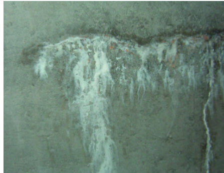
Figur 32: Kalkutvasking (lime leaching) [31]
