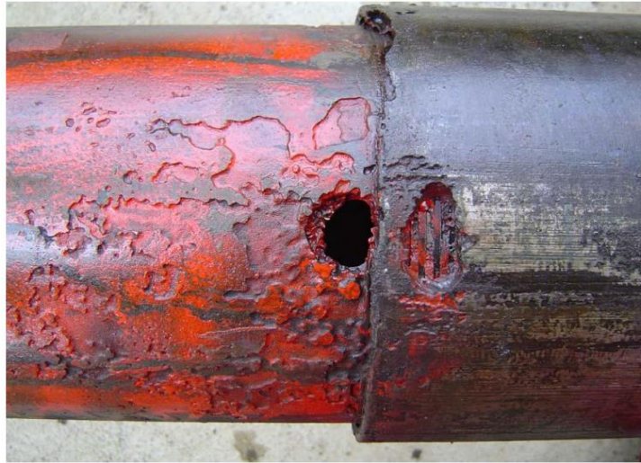
Figure 4.23: Large hole in production tubing – The leak has started at the connection and likely developed due to both corrosion and erosion (NOROG, 2012).
