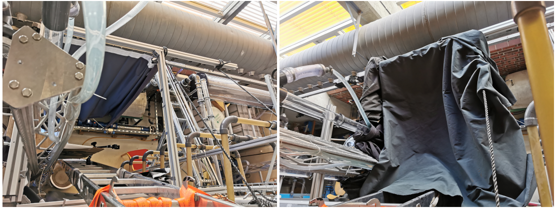
Figure D.4: Top of new setup. Curtains laying on top of new metal frame
