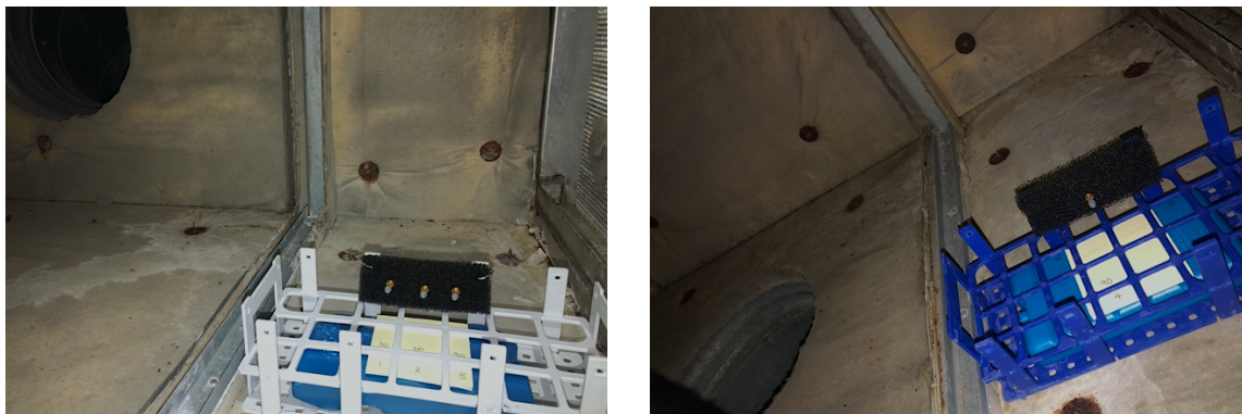
Figures 9A and B: Setup of sampling systems inside of the ventilation shafts of room 11 (left) and room 12 (right). Air flows from the hole and continues through the filter at the right of both photos. SPME fibres were fixed through a piece of mesh to keep them perpendicular to the air trajectory.
