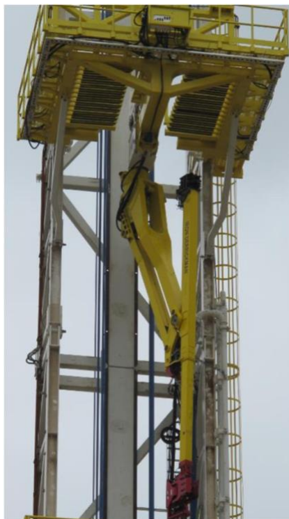
Figure 2-8. Automated pipe handling system [26]
