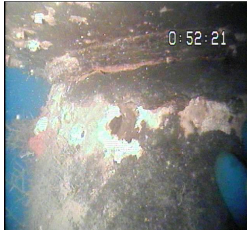
Fig 2.6: fatigue damage of horizontal member of East Cameron Area platform (ENERGO May 2007).
