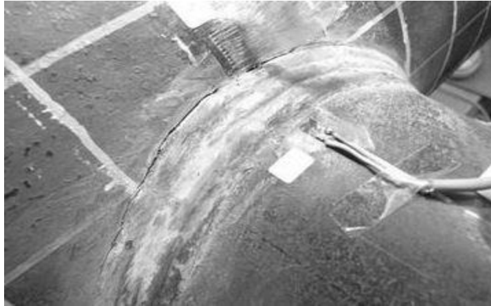
Fig 5.24: shallow crack at the weld toe.
