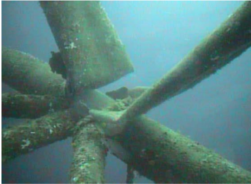
Fig 5.19: damage of joints from MMS project (ENERGO May 2007)
