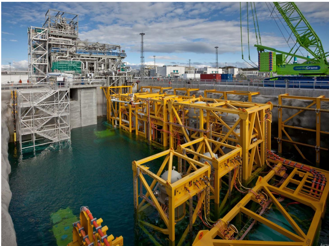
Figure 3-2 Compressor unit from the Ormen Lange field in the Nyhama basin on the commissioning phase [9].
