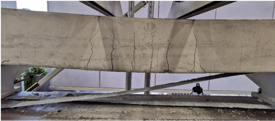
Figure 4.5 B.4 Debonded CFRP plates
