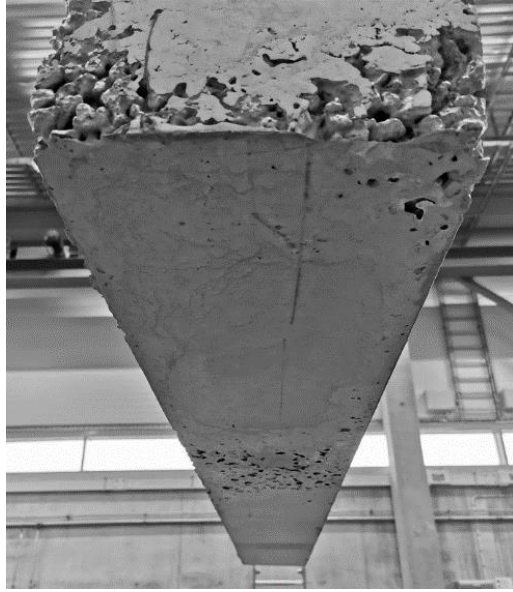
Figure 3.10 Honeycomb, tension side beam A.6
