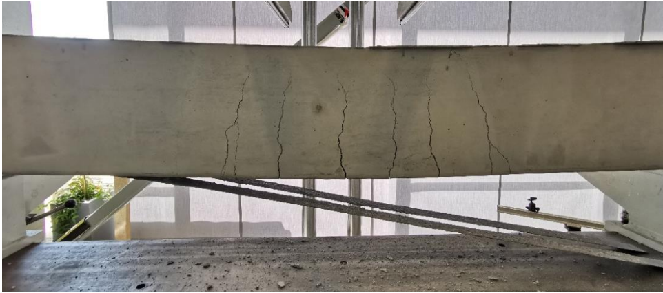
Figure 4.4 B.5 Debonded CFRP plates
