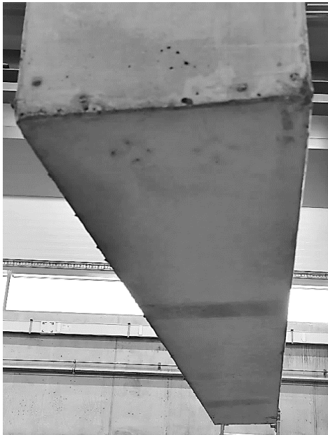
Figure 3.11 Tension side beam A.5
