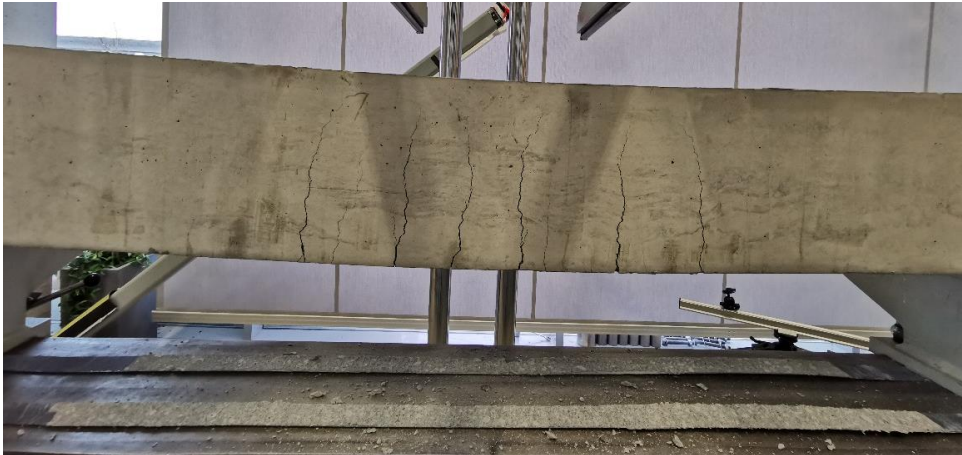
Figure 4.6 B.6 Debonded CRFP plates
