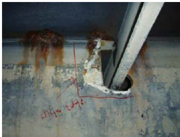
Picture 45 Marked area needs renewal. (Clipper Skagen 2009)
