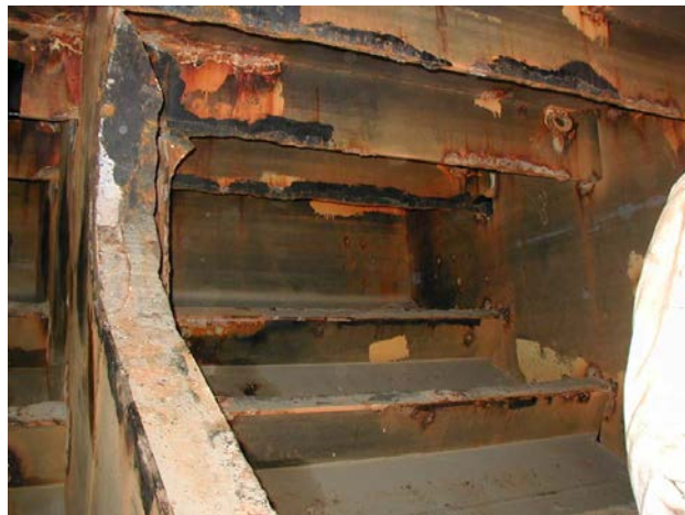
Picture 39 Coating in poor condition (IACS 2006)
