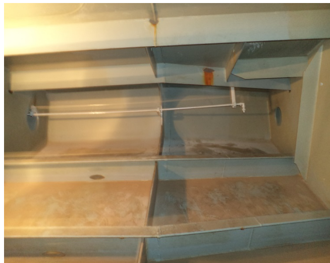
Picture 77 Corrosion in drain holes under deckhead (Clipper Mars 2013)
