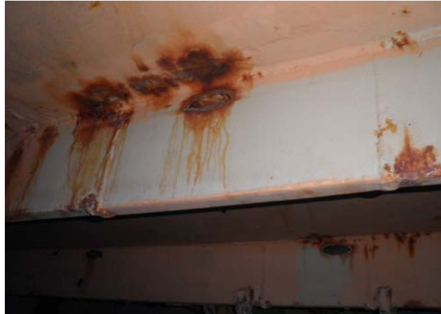
Picture 50 Corrosion on renewed steel (Ask 2014a)
