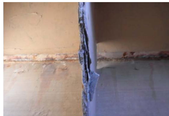
Picture 16 Rust jacking (Ask 2014a)
