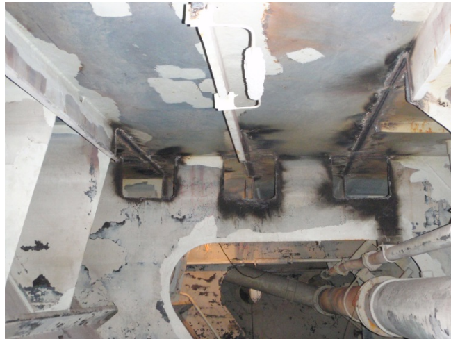
Picture 46 Corroded part cut out (Clipper Skagen 2009)
