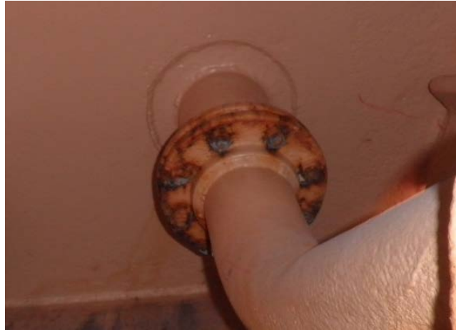
Picture 2 Corroded bolts and nuts on a flange in ballast tank (Ask 2014a)
