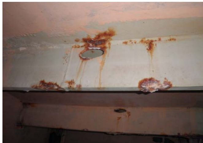
Picture 49 Corrosion on renewed steel (Ask 2014a)
