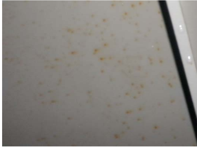
Picture 90 Pitting/abrasive dust in the deckhead (Ask 2014c)
