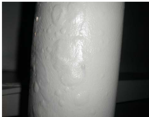
Picture 92 Blisters on a ballast water pipe (Ask 2014c)
