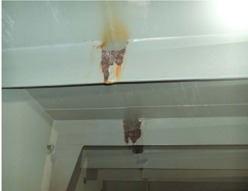
Picture 78 Drain holes in the deckhead (Clipper Mars 2014)
