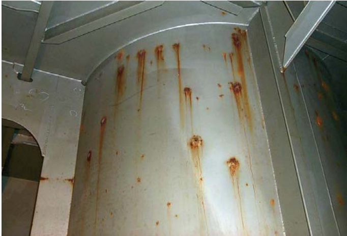
Picture 32 1% Scattered coating failure (ABS 2007)
