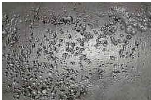
Picture 5 Pitting corrosion (NDT 2002)
