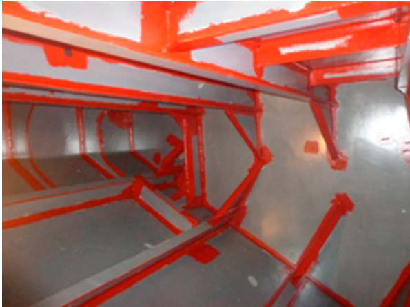
Picture 17 Stripe coated ballast tank (GS 2014)
