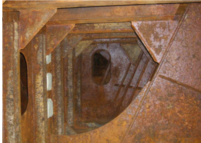
Picture 1 General corrosion in a ballast tank (Charisma 2014)
