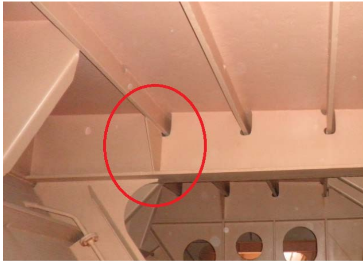
Picture 3 Stiffener support in top of a wing ballast tank
