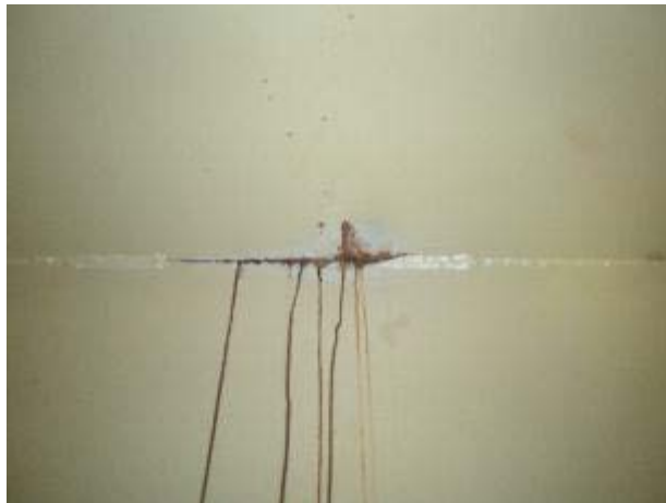
Picture 8 Crack on a weld seam (Clipper Skagen 2012)
