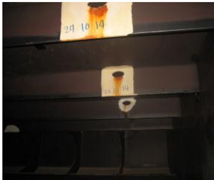
Picture 72 Corrosion in drainholes in deckhead (Clipper Star 2014)
