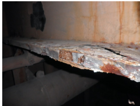
Picture 15 Rust jacking (Ask 2014a)
