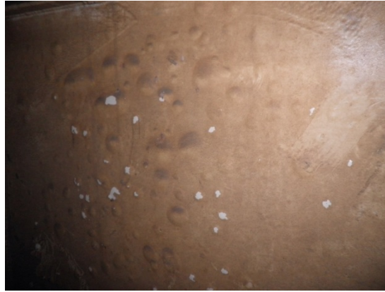
Picture 9 Small blisters in a double bottom ballast tank (Ask 2014a)
