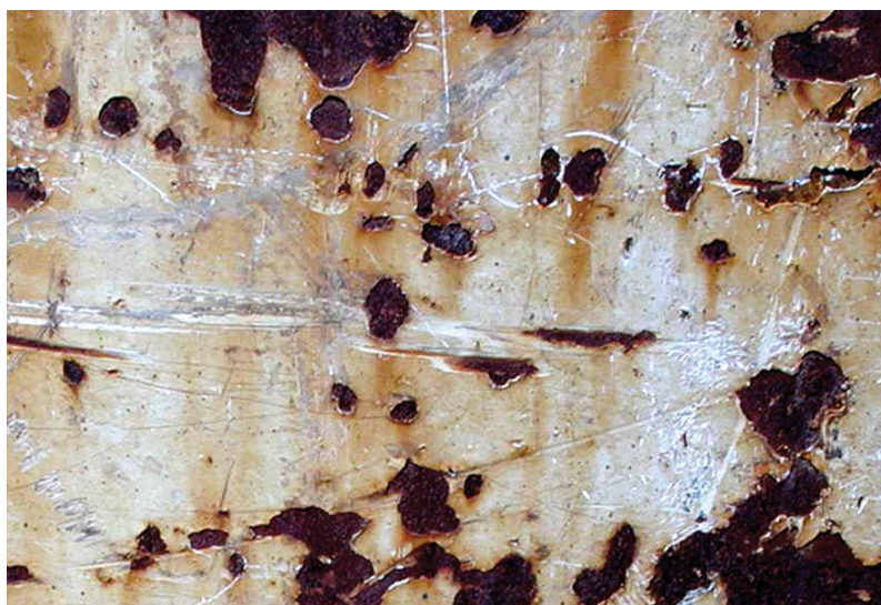
Picture 35 25% coating failure (ABS 2007)
