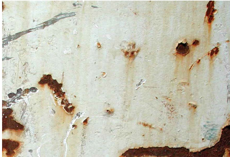
Picture 34 10% Localized failure (ABS 2007)
