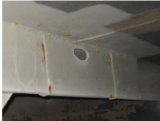
Picture 48 Drain hole one year after renewal (Clipper Skagen 2010)
