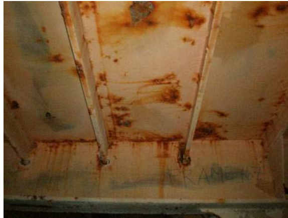
Picture 52 Before grit blasting and recoating (Clipper Skagen 2012)
