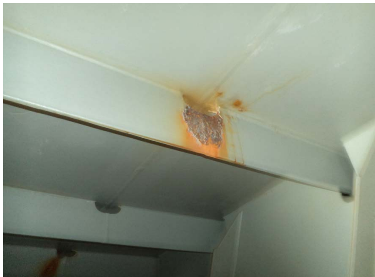
Picture 79 Drain holes in the deckhead (Clipper Mars 2014)
