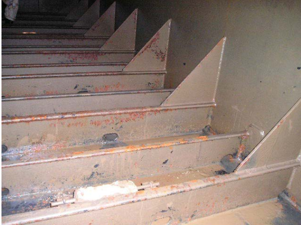
Picture 37 Coating in good condition (IACS 2006)
