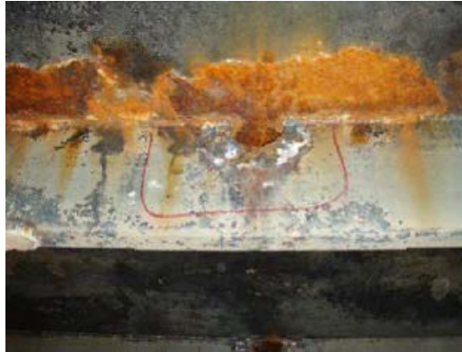
Picture 41 Edge corrosion on drain hole (Clipper Skagen 2009)
