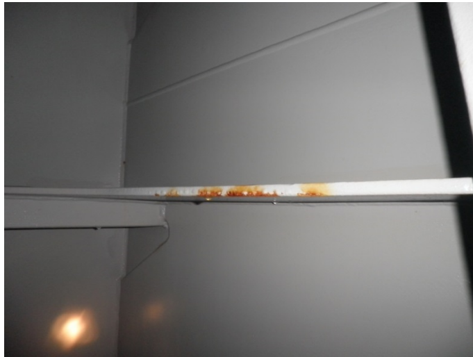
Picture 88 Edge corrosion on transverse bulkhead (Ask 2014c)
