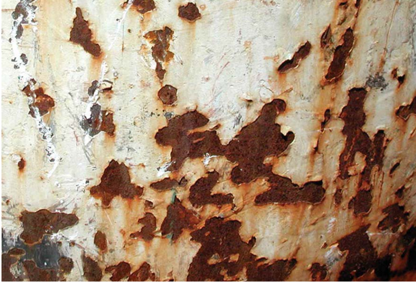
Picture 36 33% coating failure (ABS 2007)
