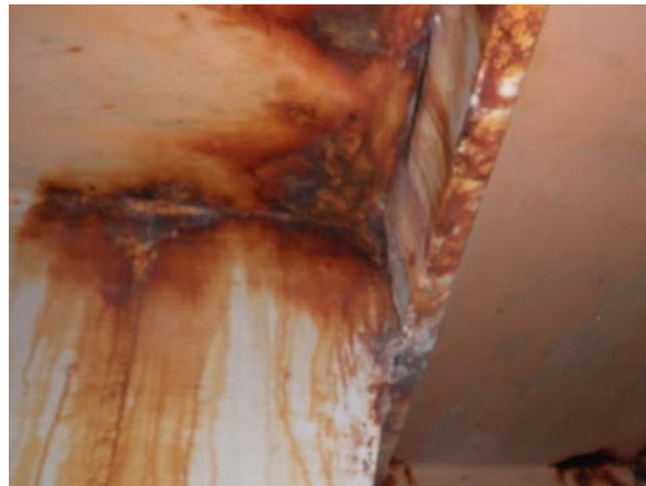
Picture 51 Corrosion near a welded insert (Ask 2014a)
