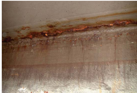
Picture 13 Type 1 weld corrosion (ABS 2007)
