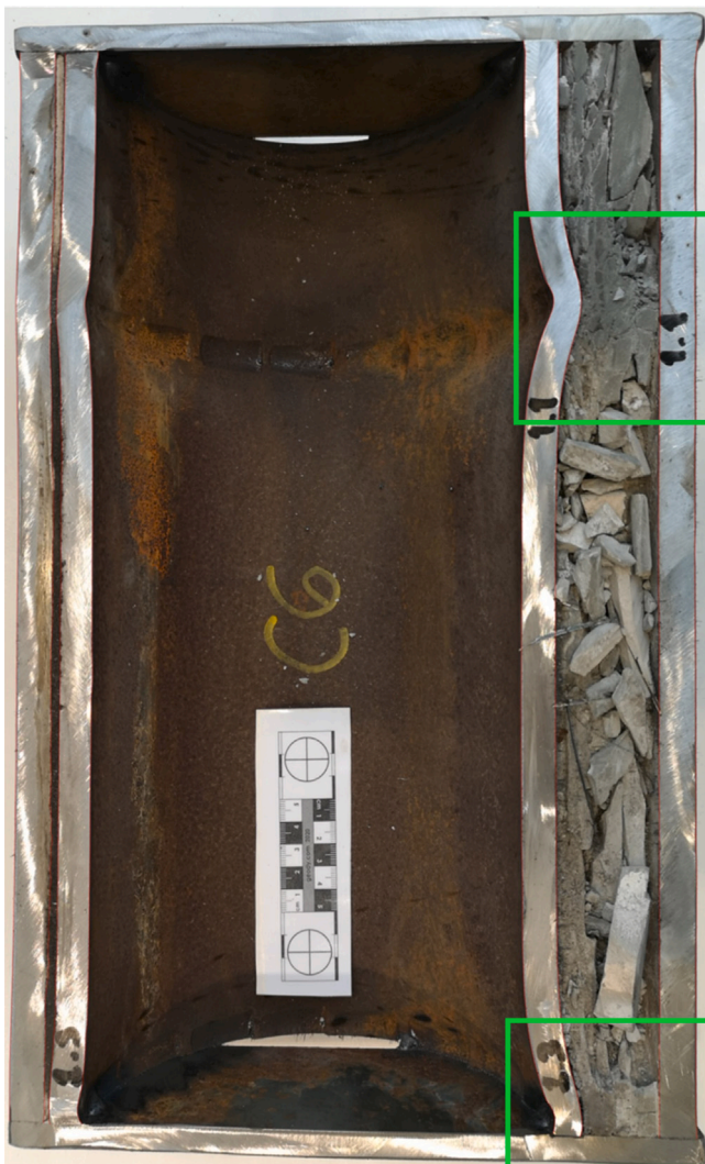
Fig. 18. Axial cross section through the dent at 1.0 m (top-most dent) and one half of the dent at 1.3 m (bottom-most dent). We observe generally fragmented and poor cement away from the dents. At 1.1 m and 1.3 m, the cement appears to have improved cohesion compared to the initial condition seen away from these positions.
