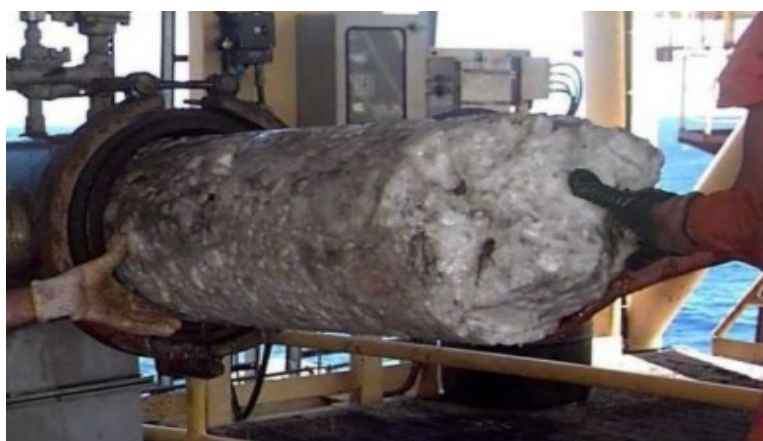
Figure 4.2. Example of a hydrate blocking the entire pipeline [24].
