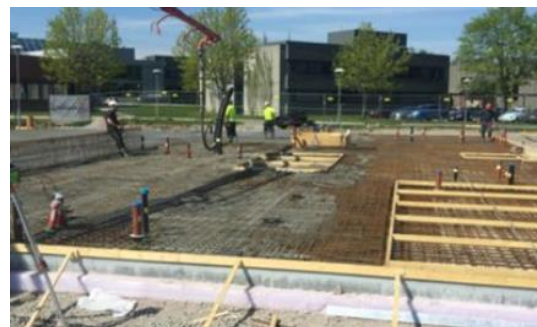
Watertight raft of the student center in Porsgrunn, Norway. 32cm steel reinforced slab with MiniBars™ to ensure crack control eliminating nets.
