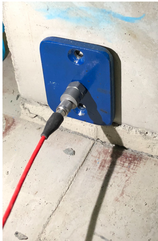
Figure 5.3. Accelerometer fastened with double sided tape
