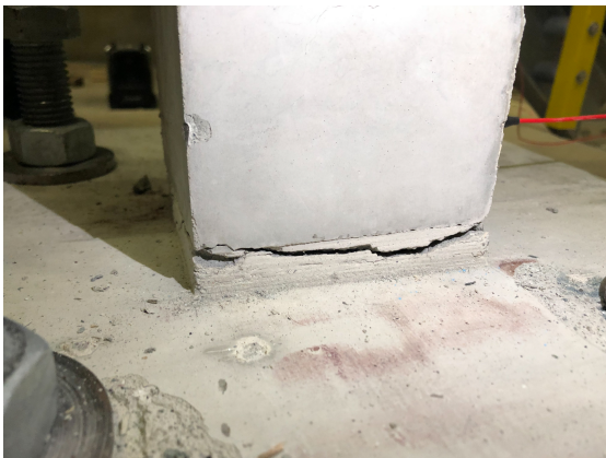
Figure 6.24. Connection crack on Specimen00
