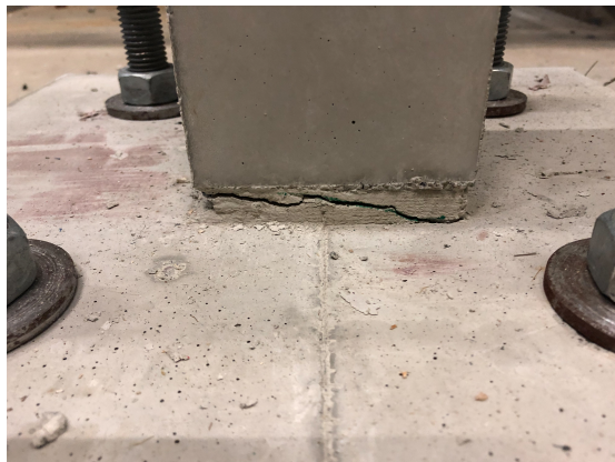
Figure 7.7. Crack formation at the footing of the column
