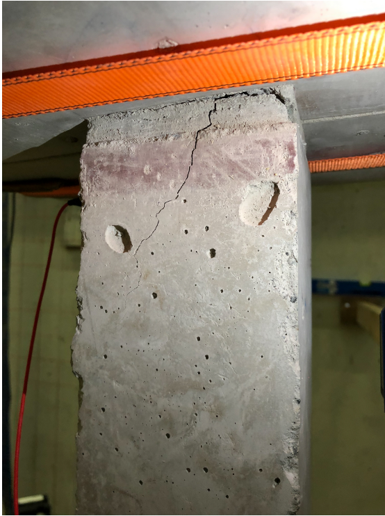
Figure 6.22. Shear crack top corner Specimen00
