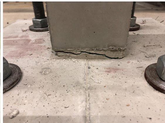
Figure 6.25. Bottom corner crack Specimen10
