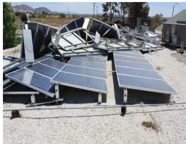
Figure 2. "Solar panel modules displaced by wind force". Credit: CASE Foresnics.(Foresnics, 2015).
