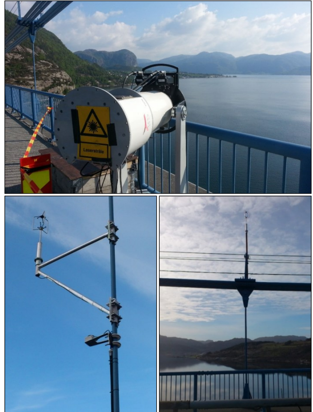
Fig. 3: WindScanner R2D1 (top) aiming at the South-West side of the Lysefjord Bridge, and sonic anemometers (bottom panels) installed above the bridge deck.
