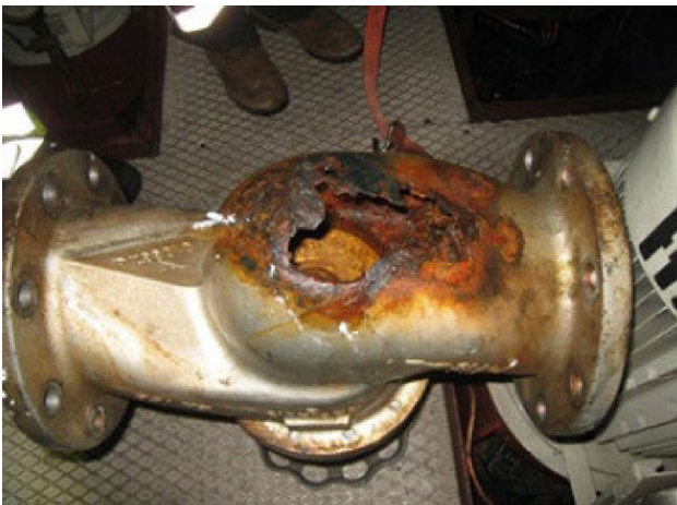
Fig. 1 Heavy corrosion on the bottom of a check valve. (Courtesy: DNV)
