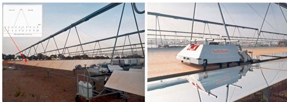
Figure 41. Dirty PV array (left) and robotic cleaning (right) [164].
