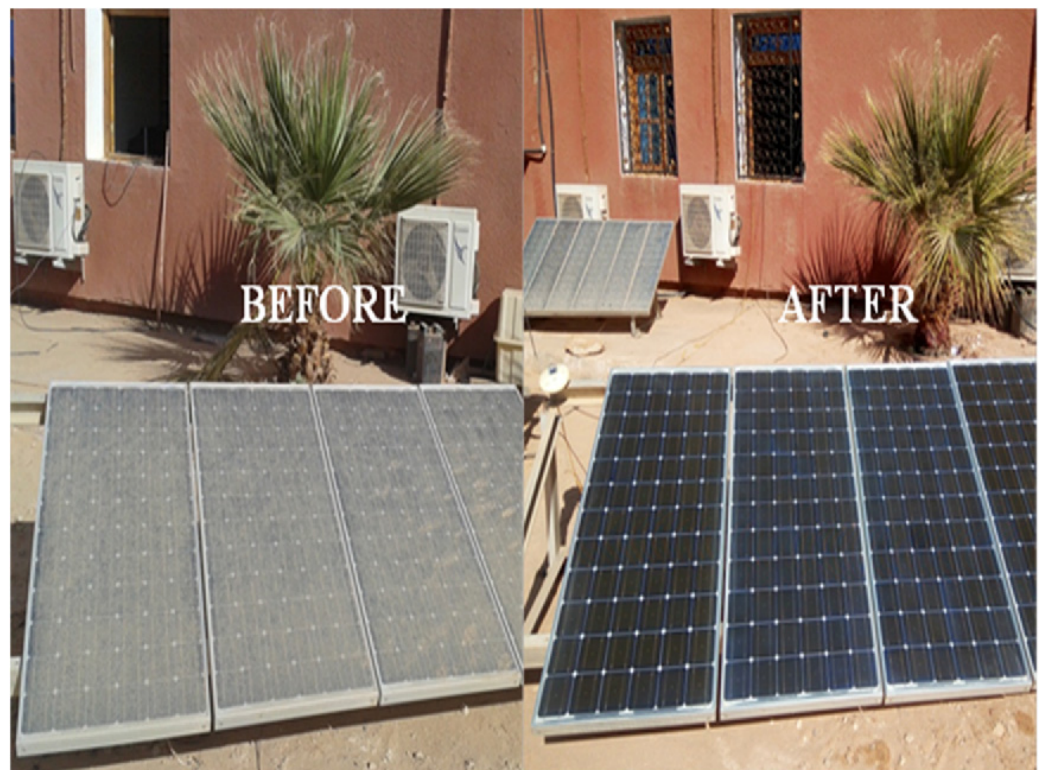
Figure 20. PV panels before cleaning and after cleaning [113].
