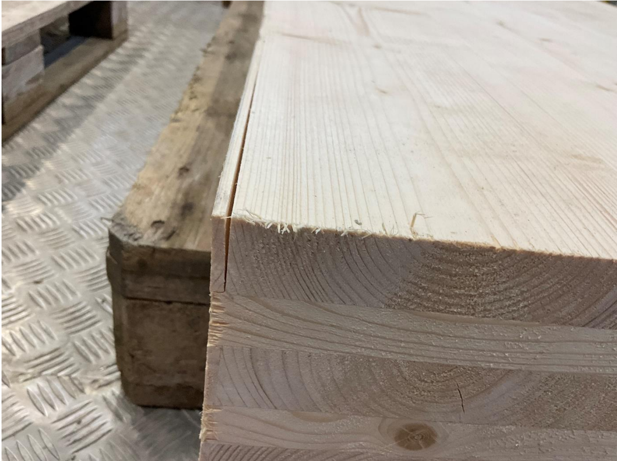
Figure 6.2 Crack observed on A2.
