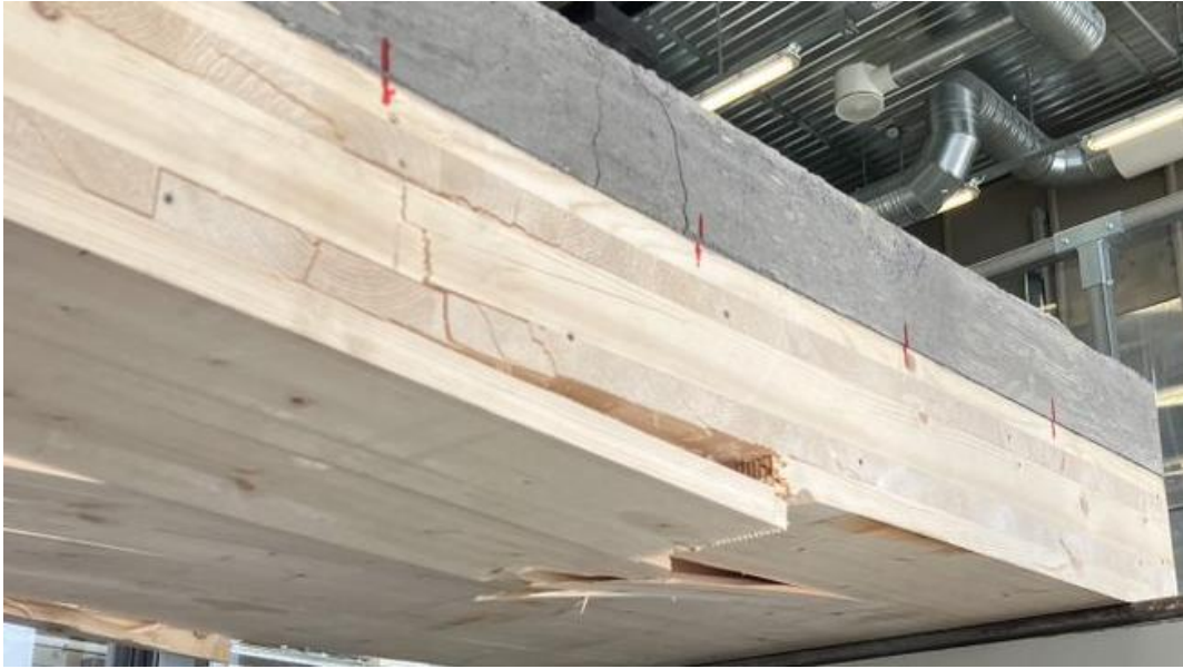
Figure 7.13 Failure of the first specimen tested (E3)
