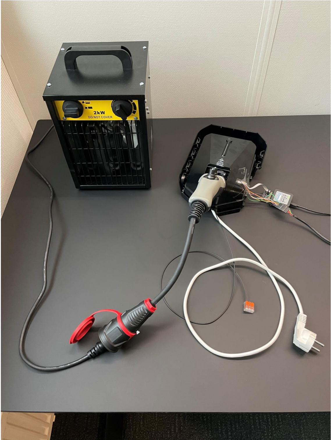
Figure 2: Finished setup for testing data collection from the charger.
