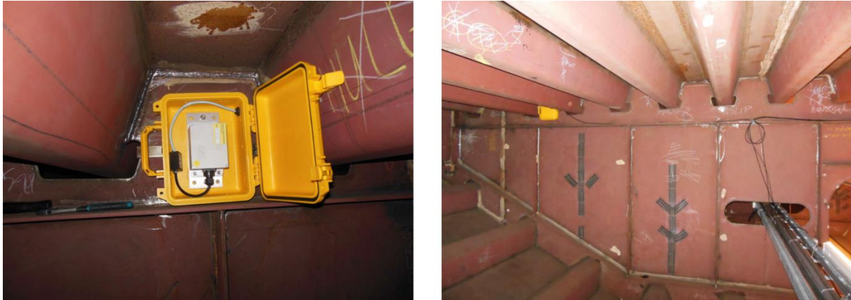
Figure 21: Accelerometer mounting position inside the bridge girder [7, p. 6]
