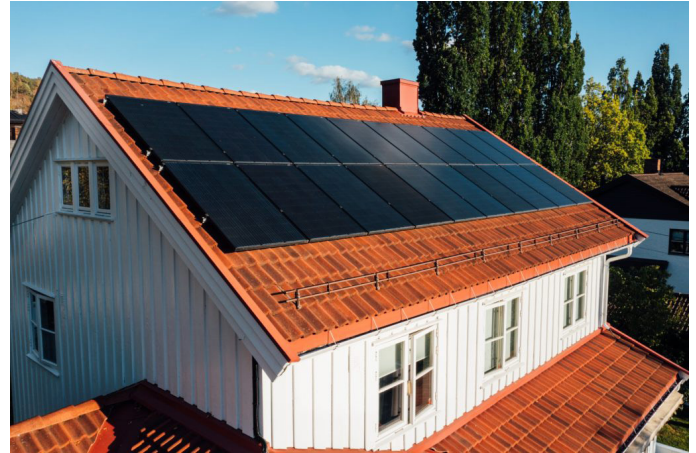
Figure 15: BAPV on a roof. ( https://www.solcellepaneler.com/solcellepanel-pa-hus/ ).
