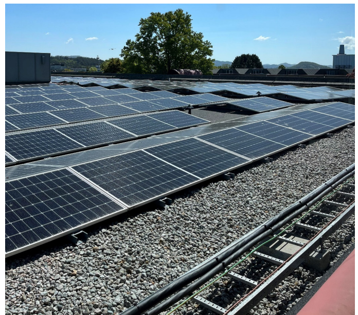
Figure 19: PV system installed on University of Stavanger roof. Own Illustration.
