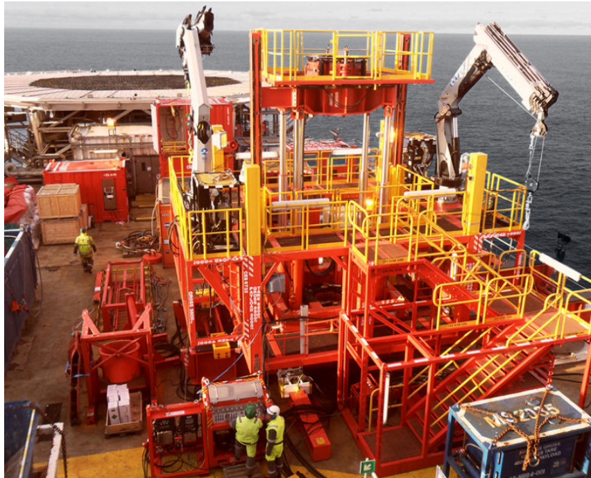
Figure 9 – Wellraizer on a wellhead platform [19]
