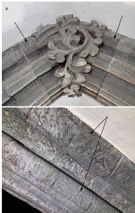
Figure 6. Tar used as an adhesive for large blocks of soapstone in the choir's vaulted ceiling. Arrows indicate stones adhered with tar. Photo: Bettina Ebert, Museum of Archaeology, UiS
