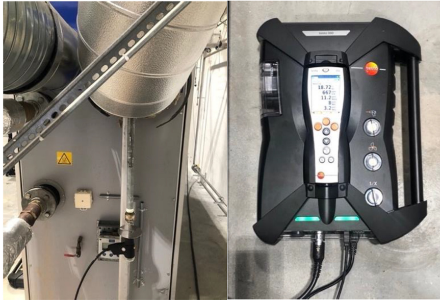
Fig. 15 – Exhaust gas composition measurements, probe installed on exhaust path in the left and analysing kit in the right.
