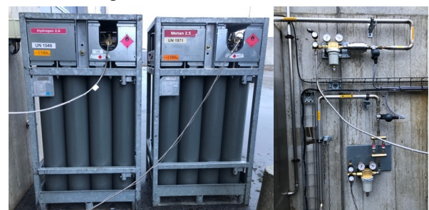
FIGURE 2: HYDROGEN AND METHANE FUEL BUNDLES AND VALVES
