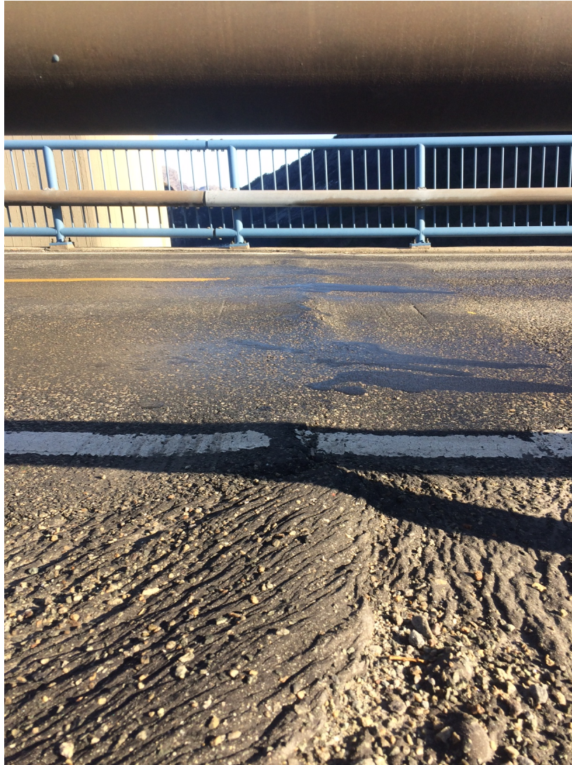
Figure 3.27: Bump in pavement by entrance to bridge on the South side of the bridge
