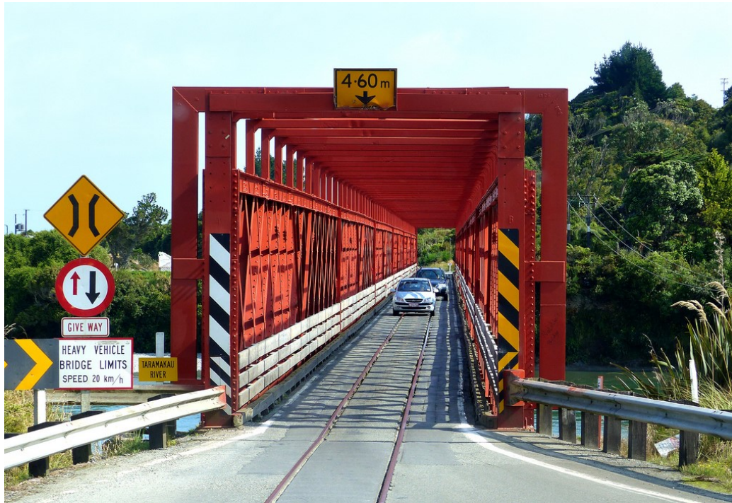
Figure 3.37: Taramakau River bridge located in New Zealand with speed limitation for heavy vehicles. Image credit: Bernard Spragg (nd)
