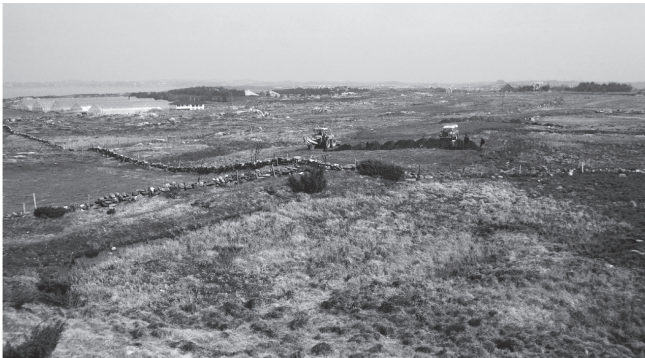
Fig. 48a. A hydraulic excavator is digging a trench through the ridgeformed structure at Jåsund, Sola municipality. Picture towards northeast (photo: Hanne Thomsen).
