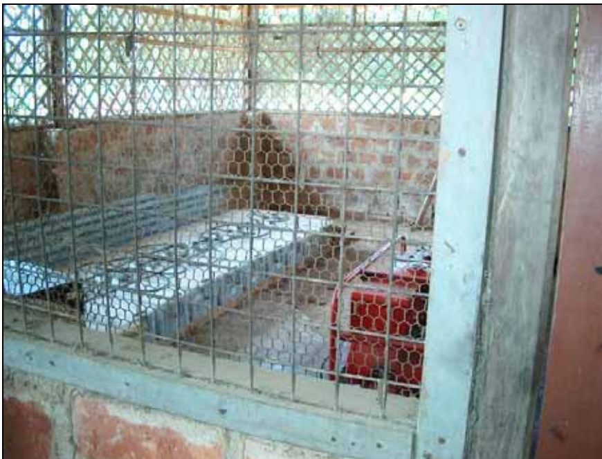
Fig. 4. Battery Storage System
