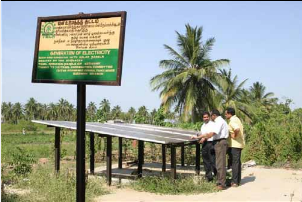
Fig. 2. Solar panel installed in NE-SL
