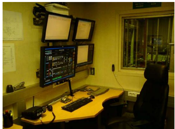
Figure 17: Inside Halliburton`s Control Cabin.
