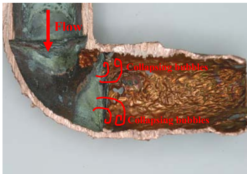
Figure 2.5. Corrosion on copper piping due to high water velocity and cavitation (Copper, 2012)
