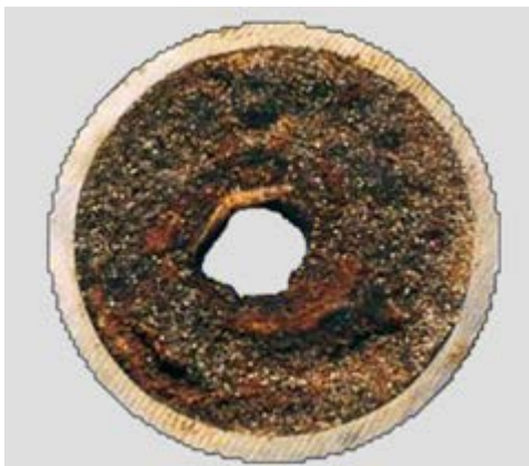
Figure 5 Wax precipitation inside pipeline wall [12].
