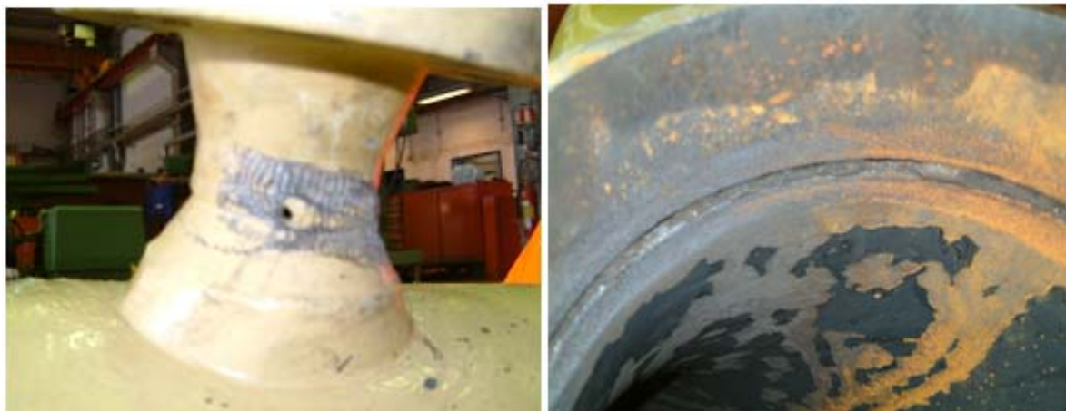
Figure 2.6.8: Corroded hole in the 2" sample point and in welding of 10" pipe (Gassco)
