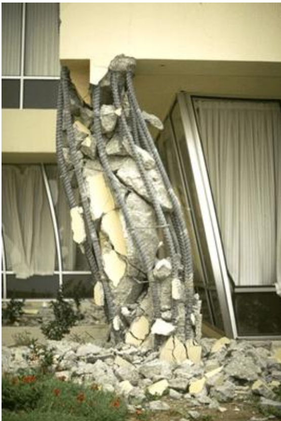
Fig 2.11: Fractured column of the Olive View Hospital building. (EERI) xix
