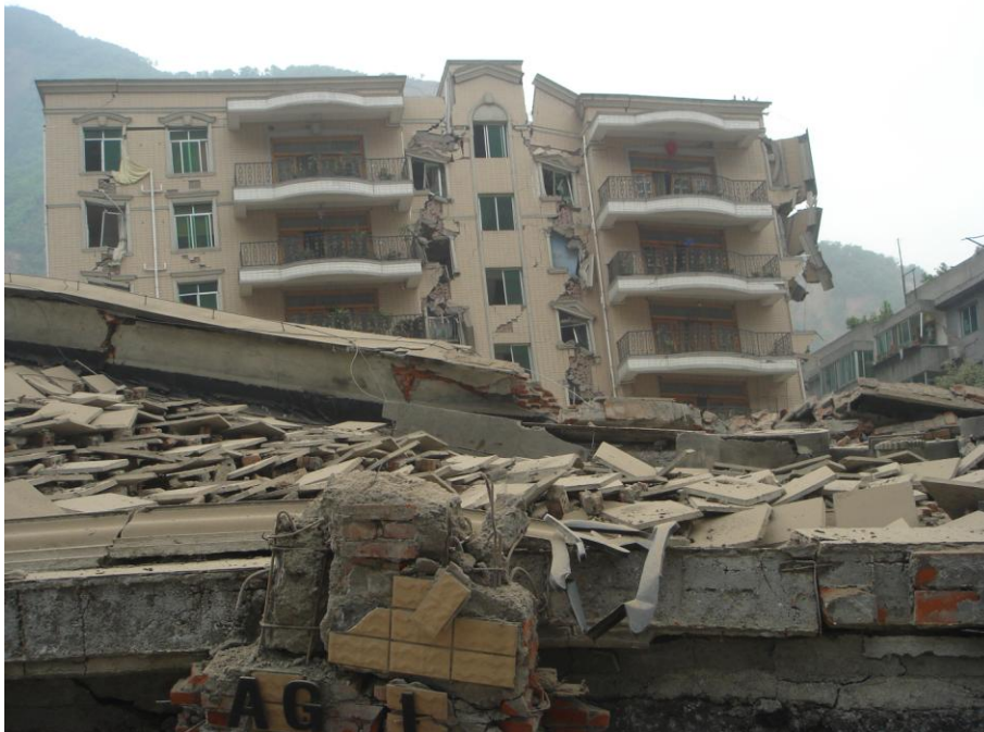
Fig. 1.3: Diagonal cracking beams and pier columns. 2008 Sichuan earthquake. (Wikipedia) iii
