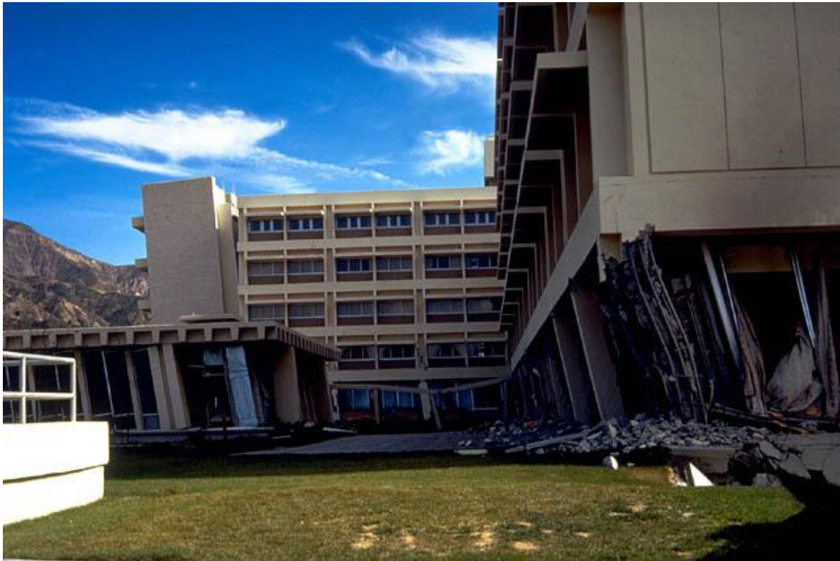
Fig. 2.10: Olive View Hospital after the San Fernando earthquake in 1971. Large deformations occurred in the first story columns. (U of C) xviii
