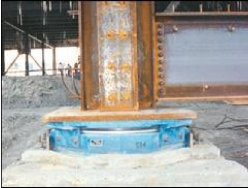
Fig. 2.15: San Francisco Airport: Friction Pendulum Bearing at base of column. xxiii
