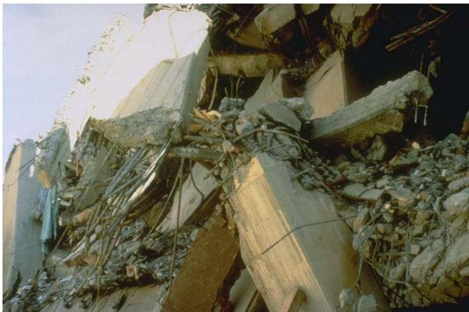
Fig. 1.2: Close-up of failed member of Juarez Hospital, 1985 Mexico City earthquake. (Western Washington University/USGS) ii
