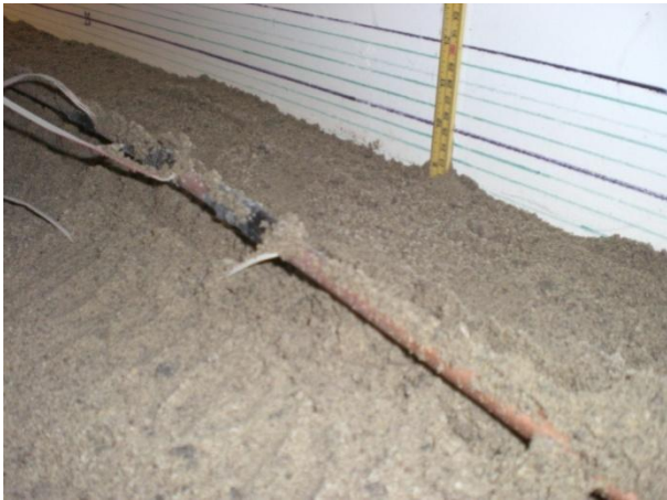
Figure 5.9 Pipe exposed after experiment and metric measurer to detect the vertical deflection.
