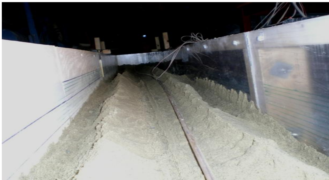
Figure 7.11 Buckling of trenched pipe
