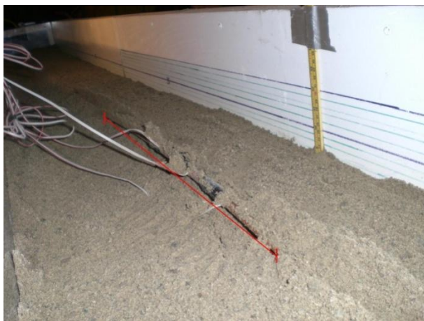
Figure 5.19 Pipe exposed post buckling
