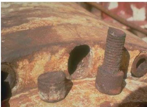
Figure 7 Detail of Failed Bolt [Upton, T.L., 2009]
