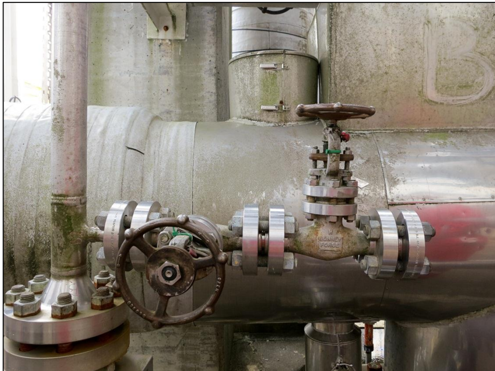
Figure 4-4 Flange Q-B-L—1100-06C connected to CA-21-5110-FS20A in area A22
