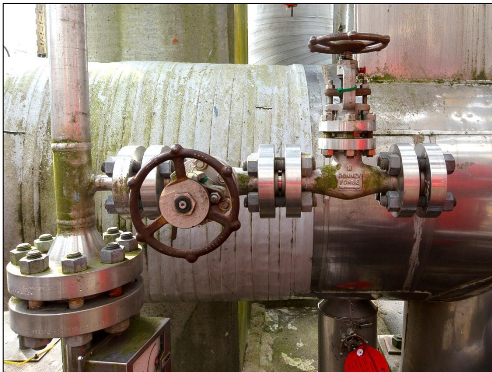
Figure 4-2 Flange Q-B-L—1100-06C connected to CA-21-5111-FS20A in area A21
