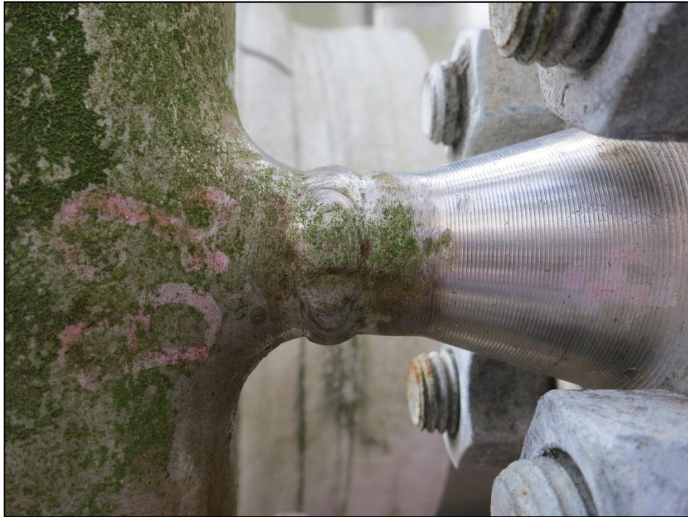
Figure 4-5 Detail of socket connected to CA-21-5110-FS20A in area A22
