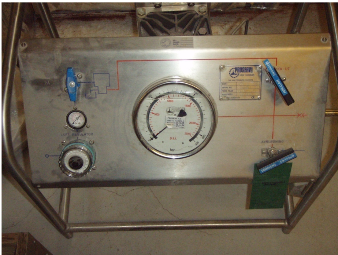
Figure 6.3: High pressure unit
