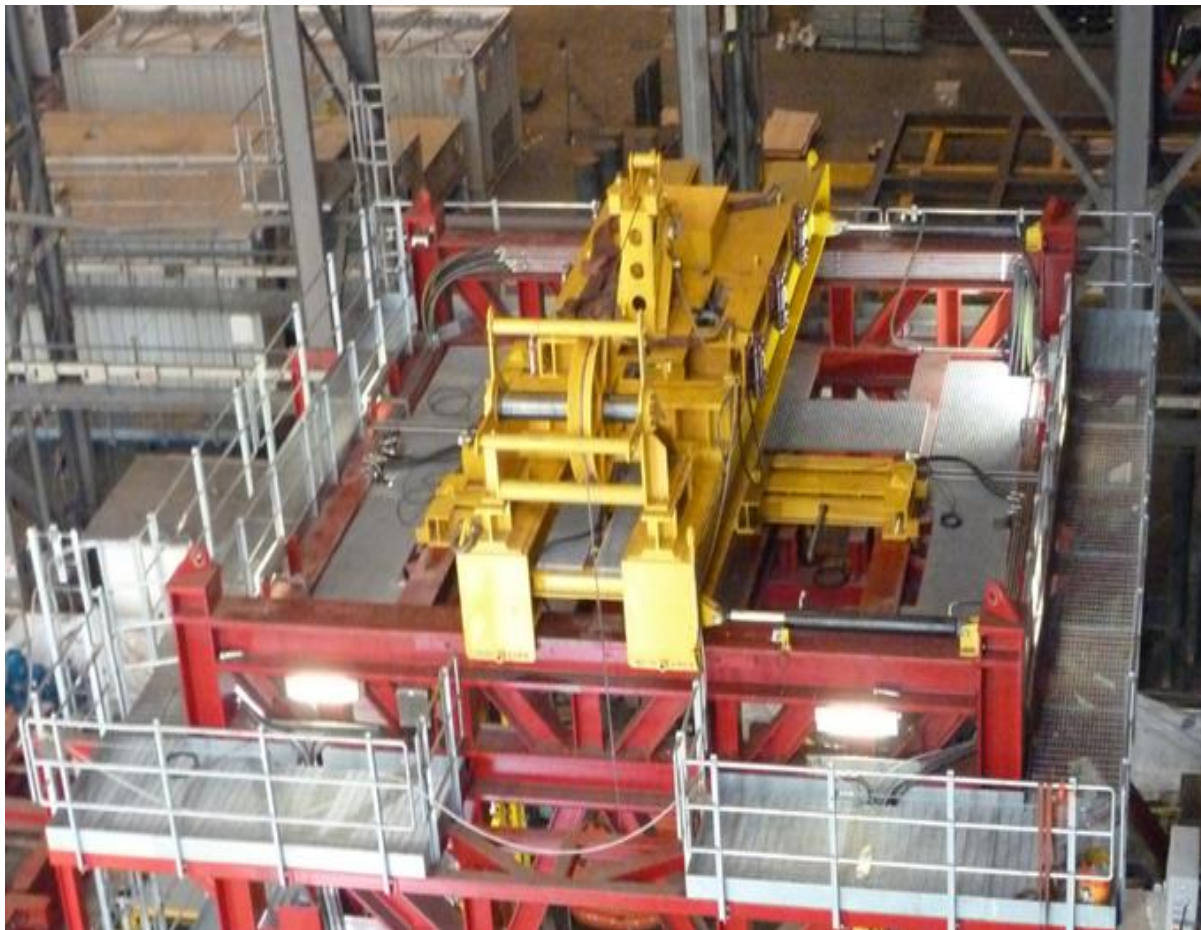
Figure 11: Main sheave assembly
