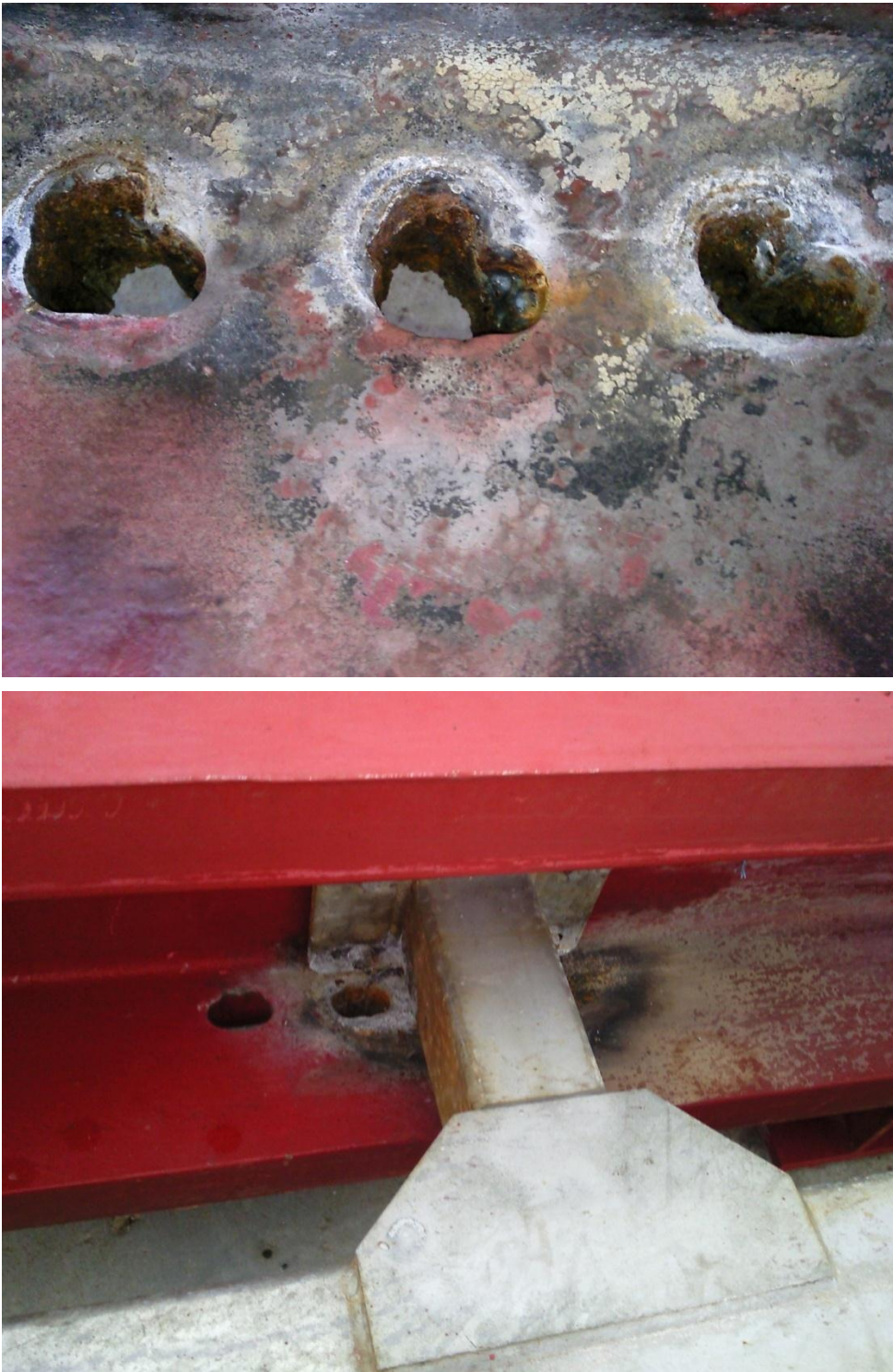
Figure 51: Burned holes in beams
