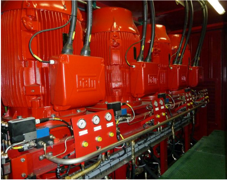
Figure 45: Motors in HPU
