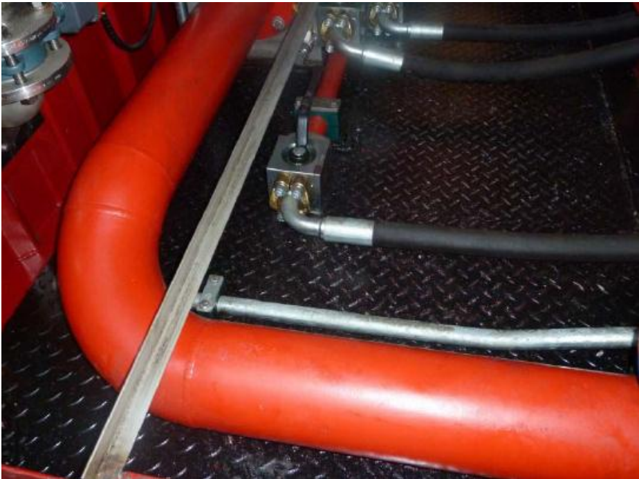
Figure 47: Oil leak on the valve
