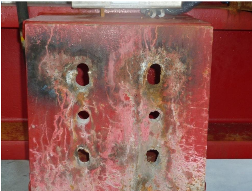
Figure 50: Bolting plate on tower for the cursor rails
