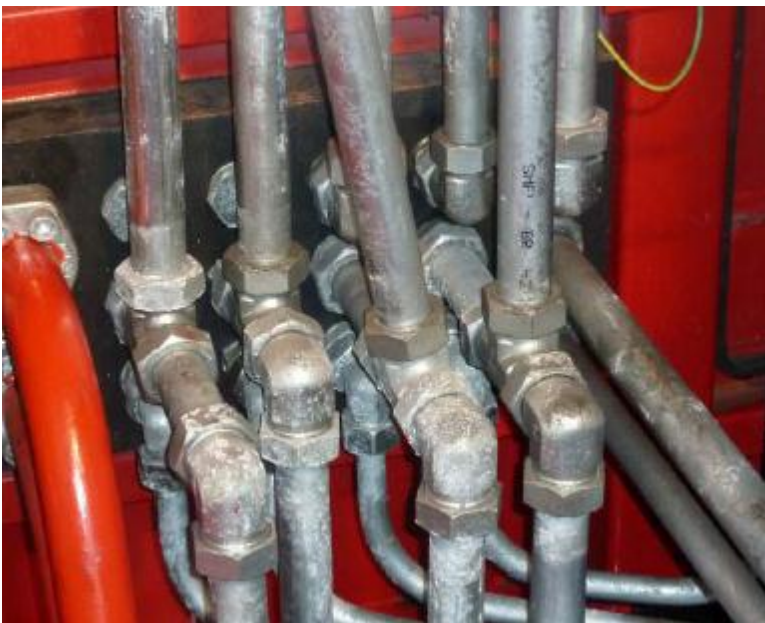
Figure 46: Corrosion inside the HPU
