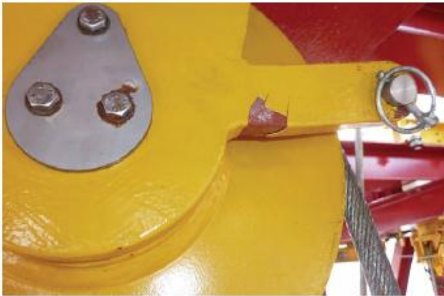
Figure 18: Damage to the sheaves
