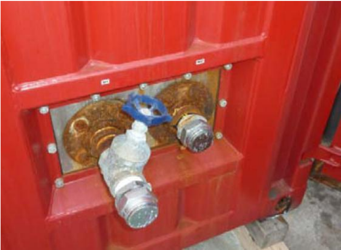
Figure 48: Corrosion in the fittings
