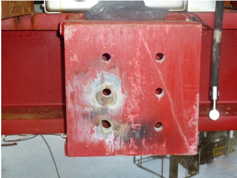
Figure 49: Bolting plate on tower for the cursor rails
