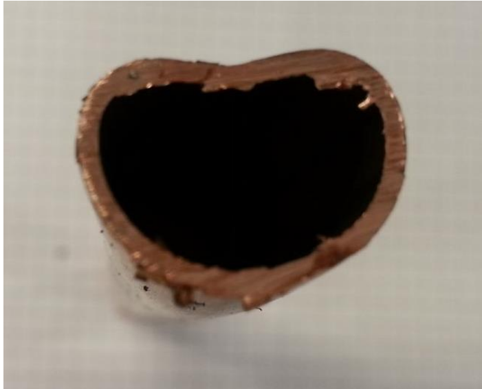
Figure 4-2 A section through a deformed pipe showing the deformed geometry
