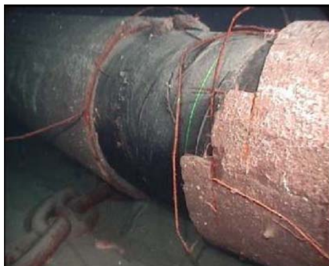
Figure 4 - Weight coat loss at damaged location 11 (Kvitebjørn gas pipe)
