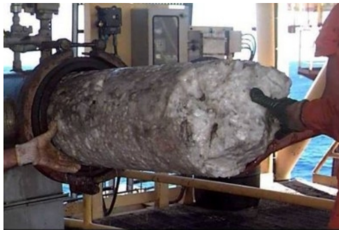
Figure 1.3-1 Hydrate plug formed in a subsea pipeline (Brazil) [95]
