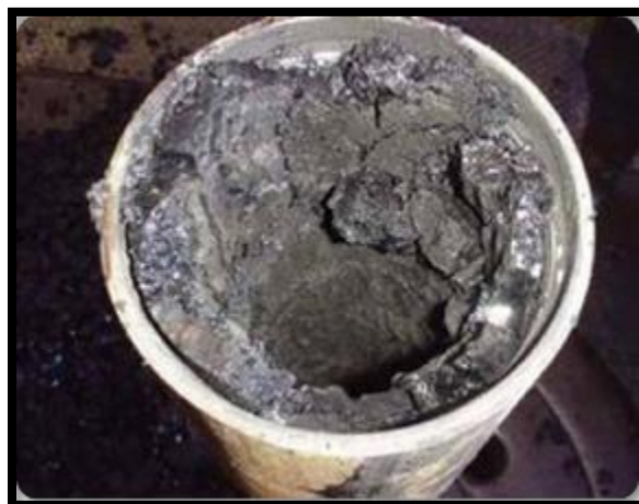
Figure 3 Picture of asphaltene deposits in a pipe (Janus Energy Resources)
