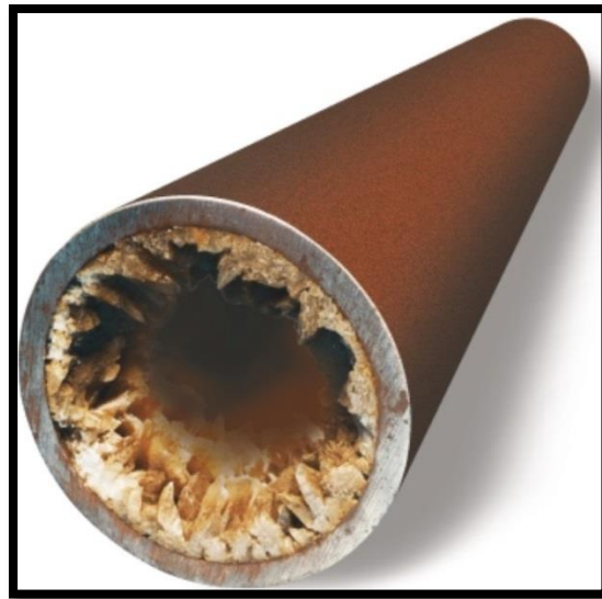
Figure 2 Pipe containing gypsum scale (Crabtree, Eslinger, Fletcher, Miller, Johnson, & King, 1999)
