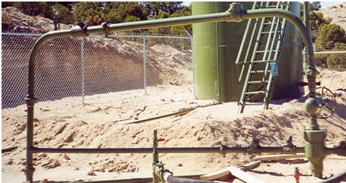
Figure 11: Shows design of pipe due to Erosion
