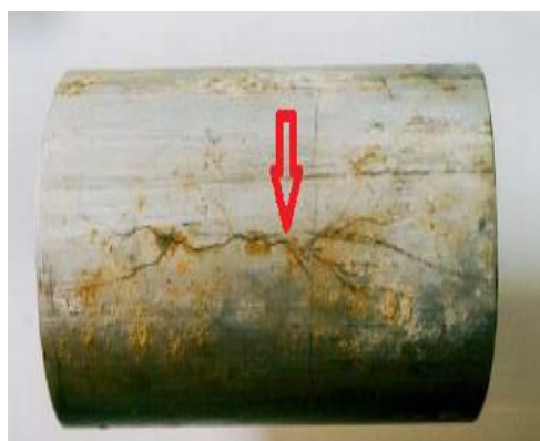
Figure 5: Stress corrosion cracking (Source-Cato Torgersen, 2012)
