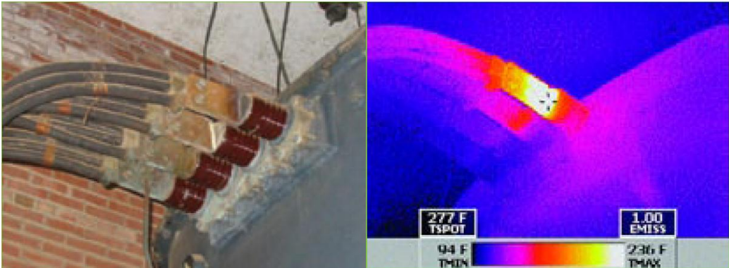
Figure 2.16 Thermal imaging of fault cable connection (Source: FLUKE Product Brochure)
