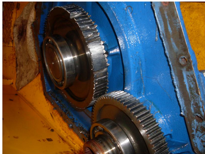
Figure 3.2 the damaged gear of Deck Crane
